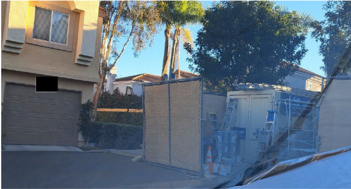
0755 hrs. rear of [REDACTED] in parking area; construction gate opened for work.
